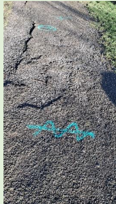
Marked for repair
